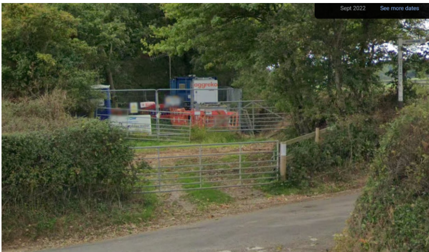
Point G looking east, showing the SWW temporary pumping station.
